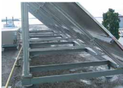
Galvanized C-channel racking system holds collector modules at optimal tilt of 45°.
