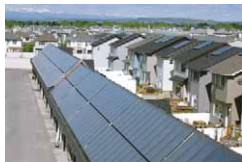
Solar collectors mounted on roofs of detached garages for district heating
