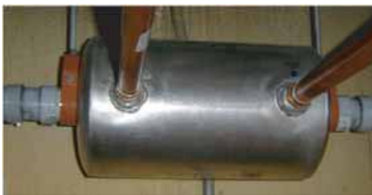
Secondary heat exchanger provides solar-heated water to seasonal outdoor pool.
