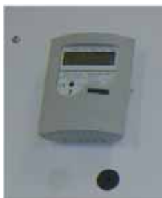
A heat meter monitors flow, temperature, and performance information, including amount of solar energy collected.
