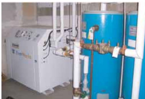
EnerWorks Commercial Energy Pack, plumbed into two 100-gallon storage tanks. Energy Pack transfers heat from collectors to water in storage tanks. Pre-heated water enters auxiliary water tanks when hot water is drawn.
