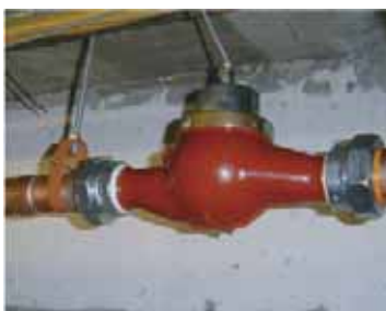
Flow meter used to determine amount of energy produced.
